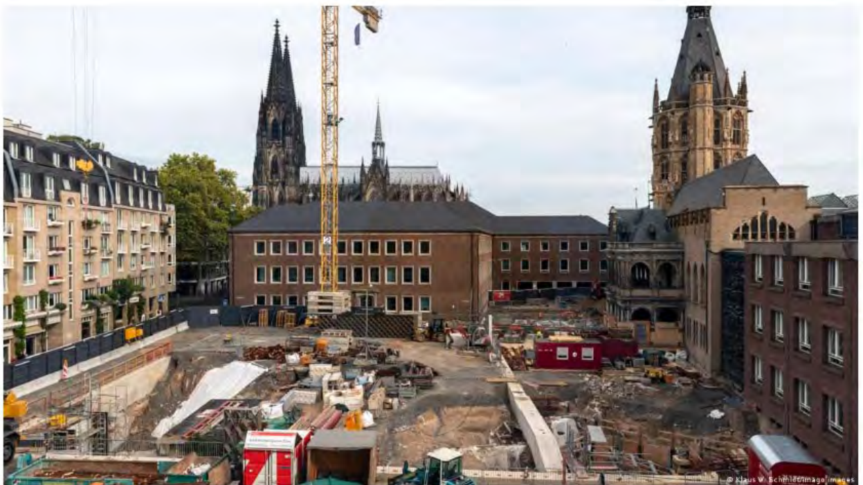
The construction of a new Jewish Museum, MIQUA, is underway in the heart of Cologne
